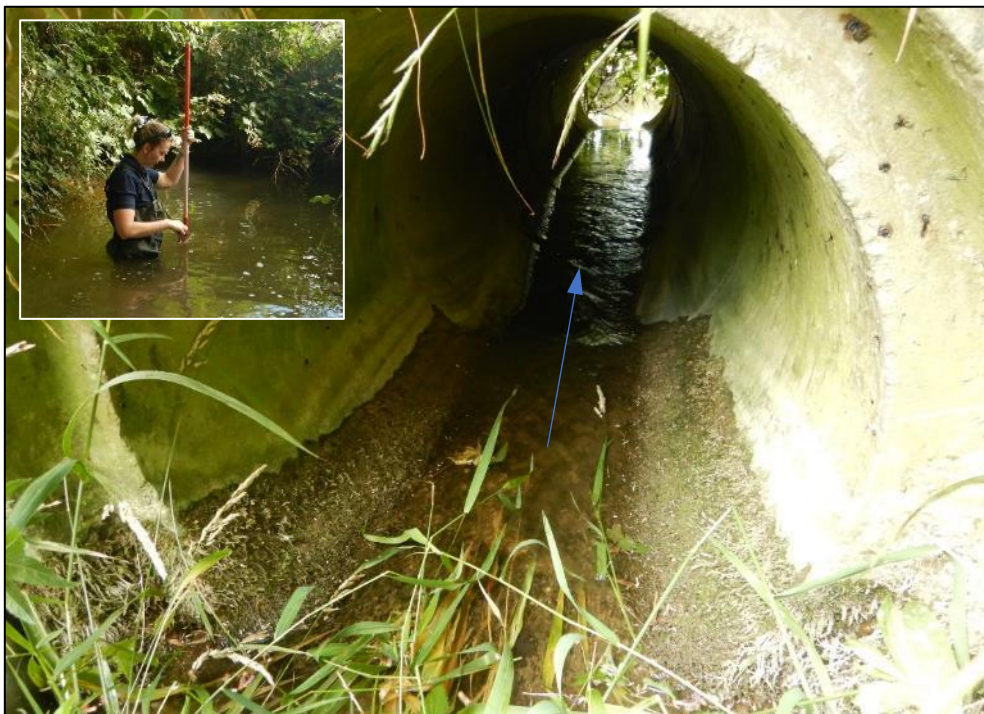
Pic 52 – Concrete culvert (0.7m diameter) creates a rapid flow into pool (0.9m depth, see inset). The shallow depth through culvert makes passage very hard in low flows. A drop \sim 0.15\text{m} occurs at the downstream end, also hindering passage. High flow would then make passage challenging as water velocity pushes fish back down the culvert. The pool is capable of holding trout but none were seen (///resonated.aside.ambitions). Trout habitat good in the pool but this culvert is likely to limit the upstream movement of trout to the reach enhanced in May 2024.
