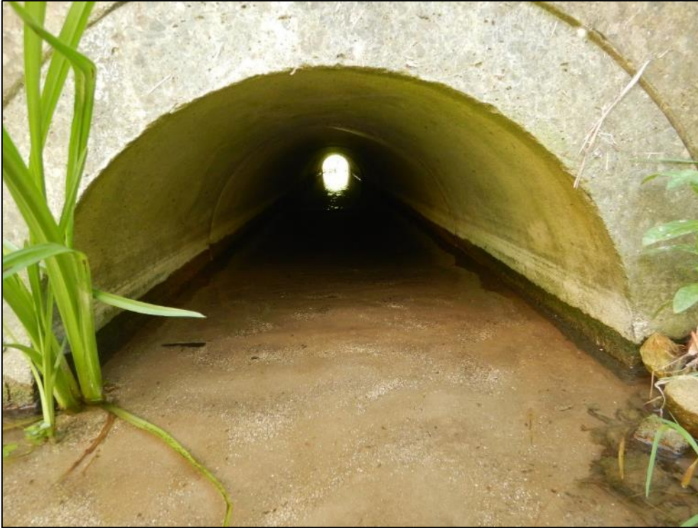
Pic 23 – The left-hand culvert (~0.7m diameter) has been set low to retain water and is almost totally silted-up making fish passage almost impossible on the day of visit (///looked.unspoiled.reliving). Trout habitat is not present.
