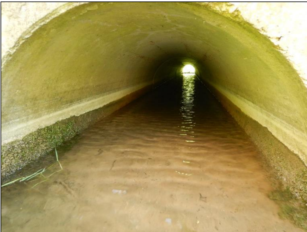
Pic 22 – The right-hand culvert (~0.7m diameter) has been set low to retain water and is partially silted-up but fish passage is still possible (///looked.unspoiled.reliving). Trout habitat is poor.
