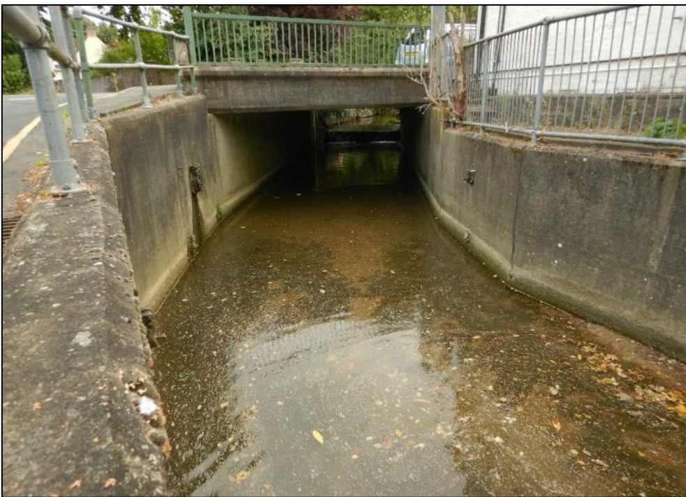
Pic 2 – Note the exceptionally poor physical habitat of the River Waring, yet fish are present. In addition to structures, poor physical habitat can present a barrier to fish migration. For example, high water temperatures and poor water quality will affect fish distribution. Note the next barrier present beyond the bridge (///majority.fats.ringside). Trout habitat is very poor.
