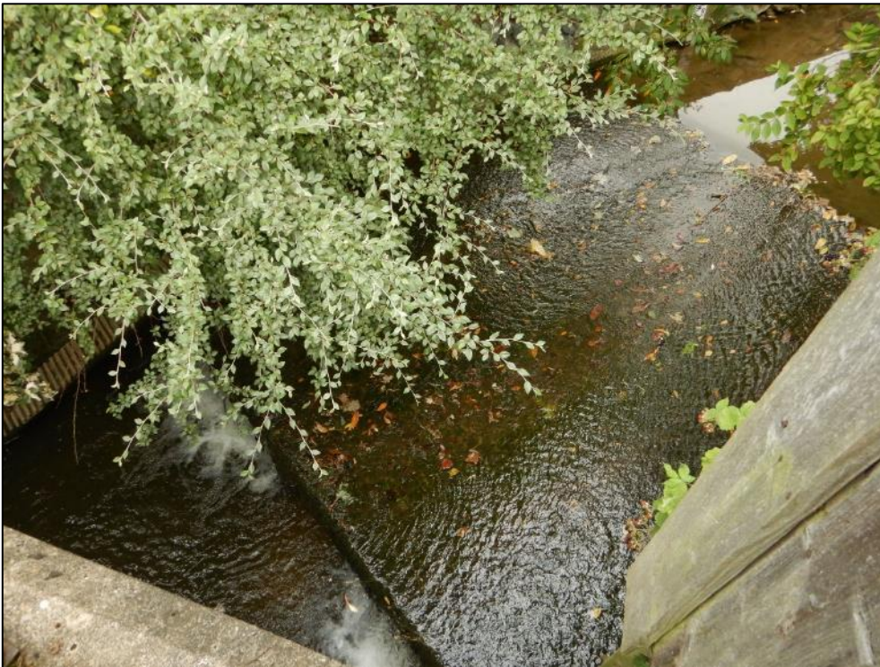
Pic 4 – The same structure as shown in pic 3 but viewed from above. A concrete spillway \sim 4\text{m} length makes it even harder for fish to traverse. In low water the depth is too low, and in higher flows the water velocity over the spillway may force fish back ( ///submerged.blaring.digs ). This structure is a significant barrier to fish migration. Trout habitat is poor.
