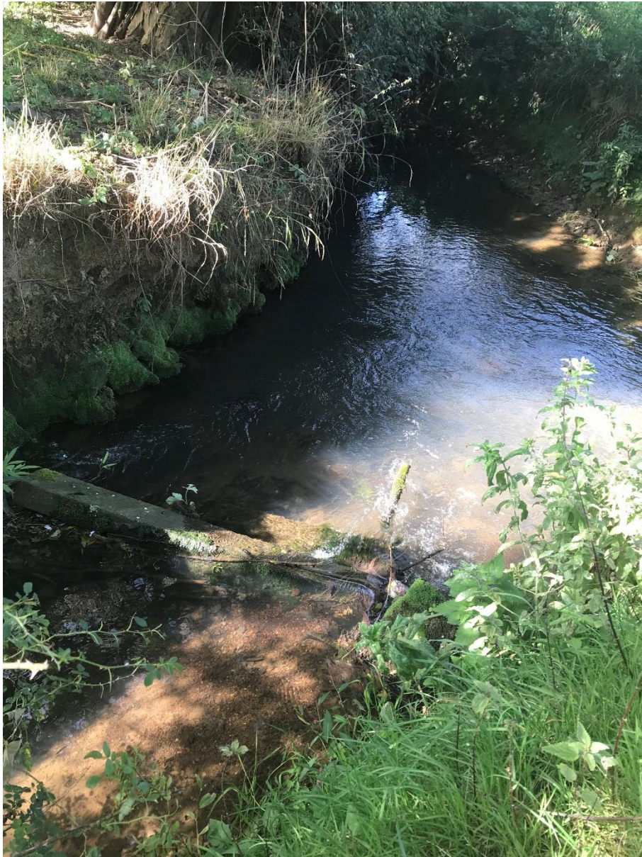
Photo 12 (52.026072 , -1.5411286) Another concrete bed check. This one is more severe with potential to impact fish migration and alter habitat upstream by artificially holding bed material back and encouraging deposition of silt. This should be removed and opportunities reviewed for introducing large woody deflectors, if appropriate. The pool habitat immediately downstream of this feature is providing additional channel variation, however the face of the RHB is bare, limiting the habitat value here. Pinning some large and brashy material here (or hinging a tree over into this location if there is one suitably adjacent) will moderate rates of bank erosion and provide some excellent habitats for fish and invertebrates.
