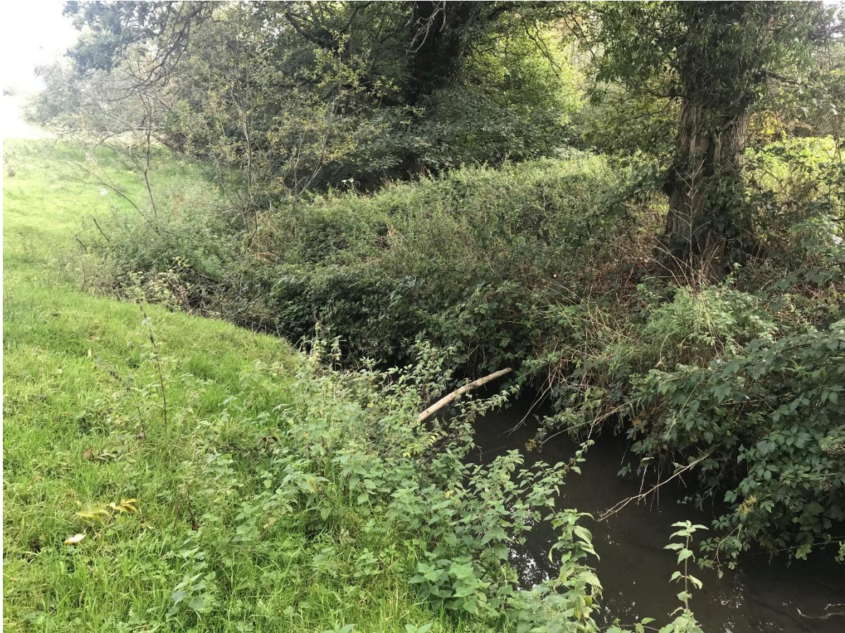
Photo 1 (52.025990 , -1.5390821) The channel around the upstream extent of the upper section; although the channel meanders, it has been over deepened, and the channel incised following drainage work.
