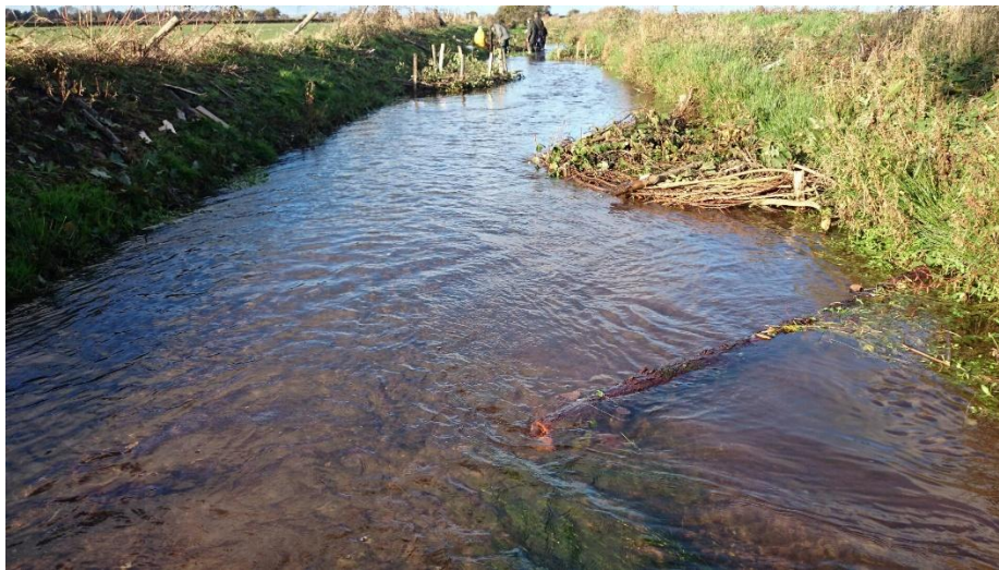
Figure 5 Features installed in a dredged channel to pinch and diversify the low flow channel. This will drive river process, encouraging the river meander.
