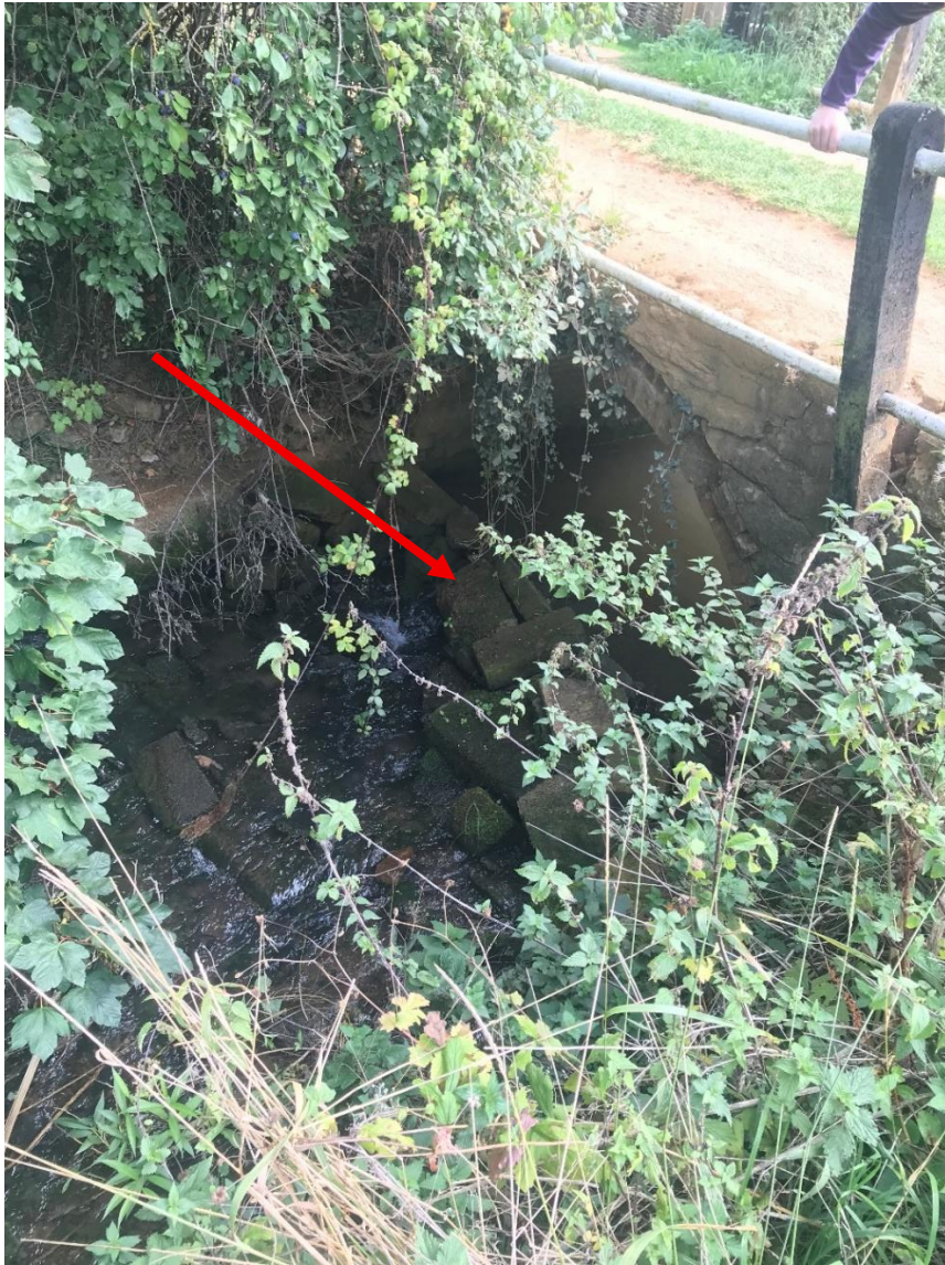
Photo 5 (52.025915 , -1.5400128) Concrete blocks have been placed across the downstream end of the access bridge arch, to hold water back (red arrow). This will be severing access for fish up and downstream and negatively altering the habitat upstream by un-naturally impounding water. If removed, the riverbed level is likely to move in the meander upstream as it re-adjusts, back up to the dipping pool. Once the riverbed 'settles' following removal of the structure, water levels can be manipulated if required for a dipping area, perhaps by using very large woody material structures, to create beneficial habitat at the same time.
