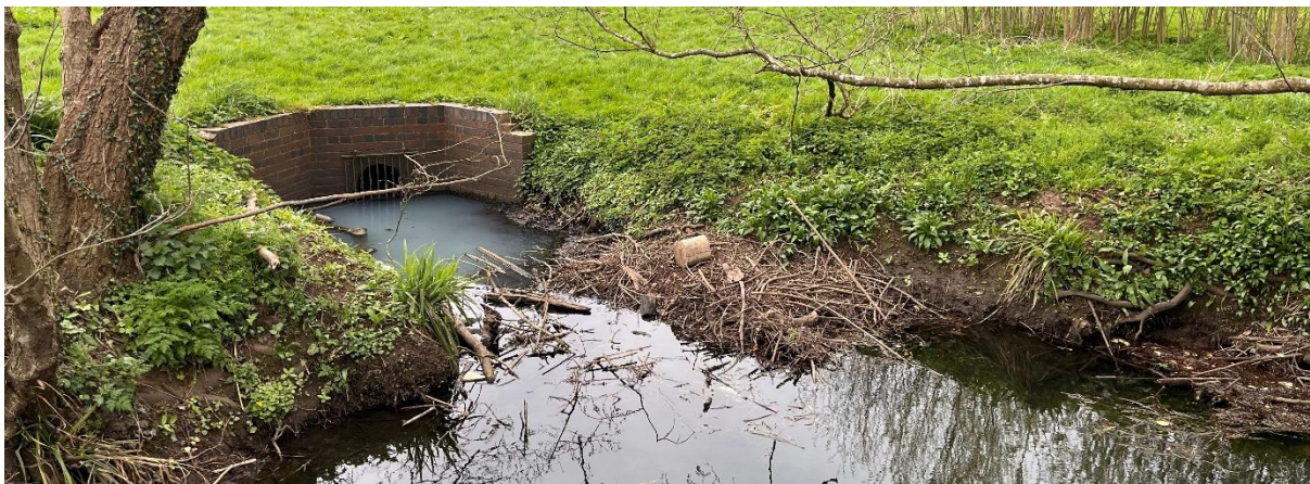
Figure 9: Probable misconnected drainage outfall at SP0391481278
