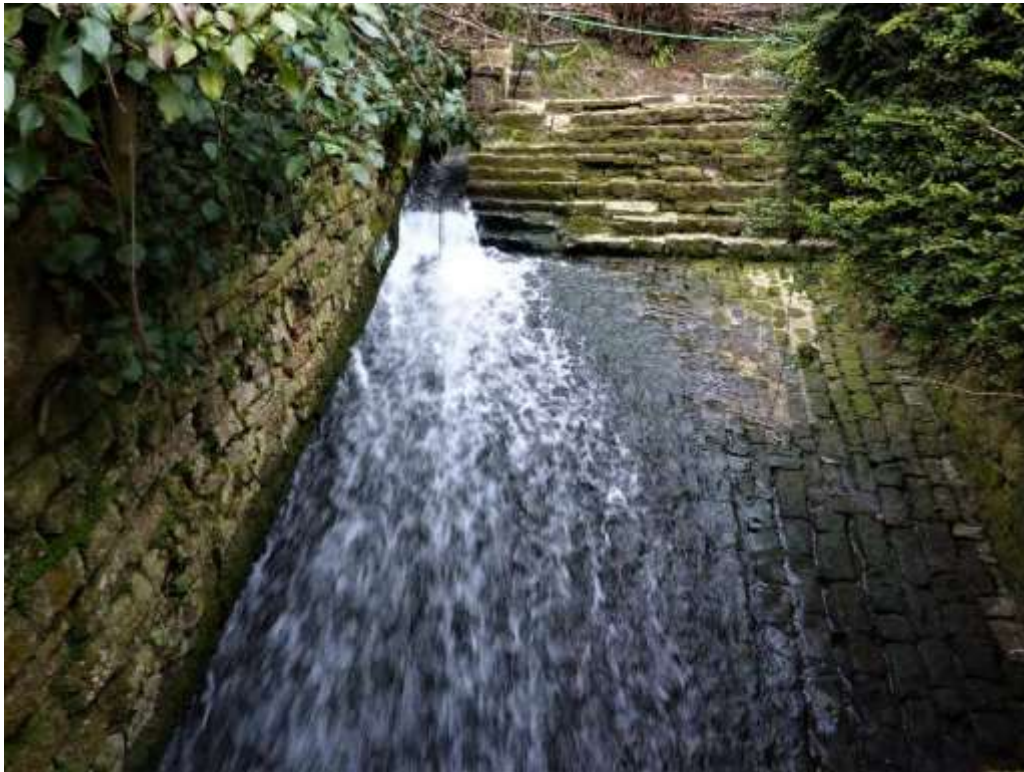
Figure 13: Shallow, impassable flow down Ham Mill weir
