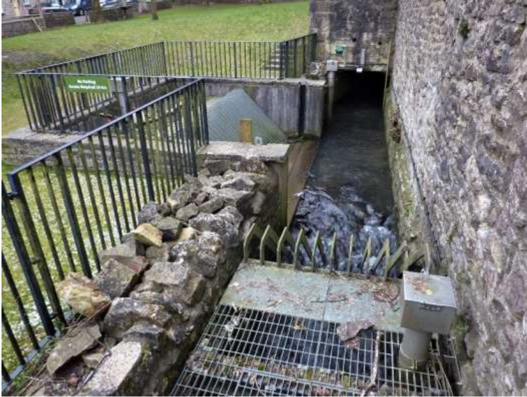
Figure 9: One of three short open culverts in the green space at the western end of Garston Street, which could be broken out as a pocket park for flood storage and social amenity
