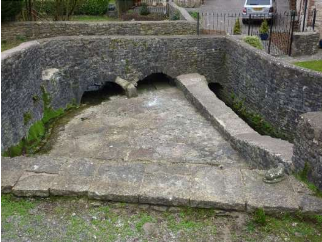
Figure 17: The complex weir structure at Darshill Mill: lower flows are presently channelled down the steep chute on the right hand side of this photo
