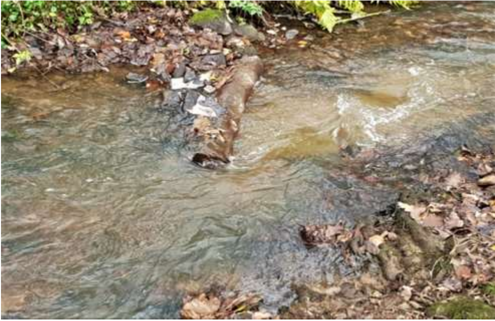
Figure 22: A flow deflector log pinned at an angle, using rebar stakes, partially across the stream (split chestnut stakes can also be used). In order to create scour in the centre of the channel, the log is angled upstream. At lower flows, the stream width is reduced, keeping the gravels clean and helping to move mobile sediment downstream. Higher flows can run over the top with little impediment.
