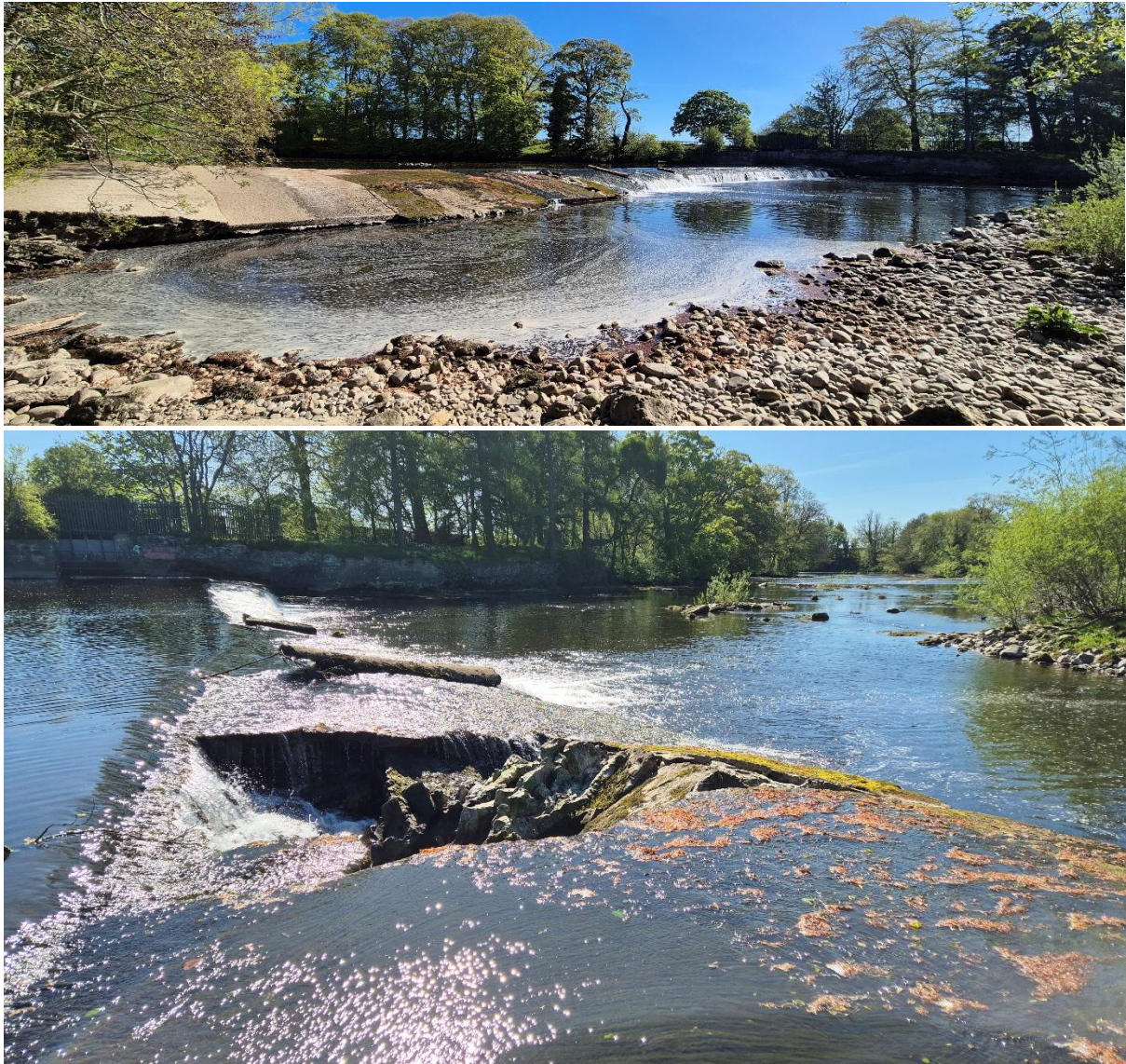
Fig 14. SE 27553 78738: Tanfield Mill weir was in a very poor state of repair, and could fail at one of several weak points under spate flow in the near future, with unknown consequences. It is a major barrier to fish passage.
