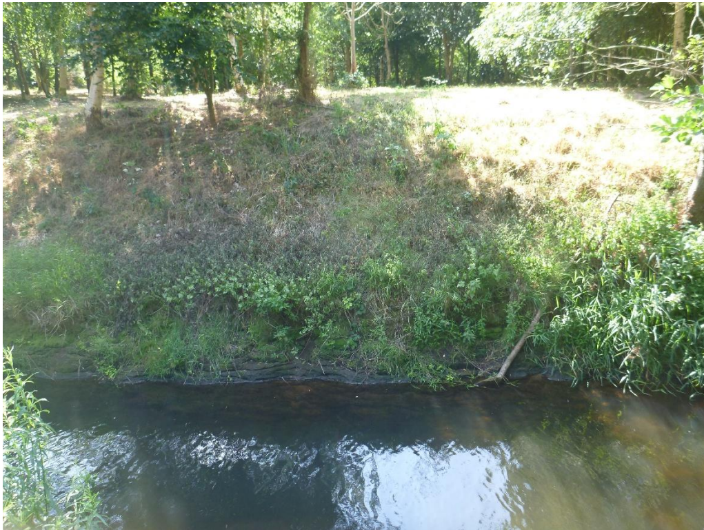
Photo 8 The steep LHB with exposed sandstone bedrock at the toe indicates the extent of channel incision throughout the reaches inspected. Despite the steepness, it appears here that the banks have been mown, possibly to facilitate canoe access.
