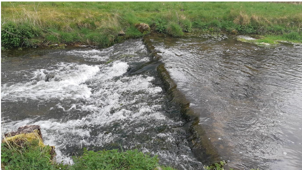
Figure 29: A low stone weir just downstream of the swimming pool weir – the small existing notch needs to be enlarged to enable free fish passage.
