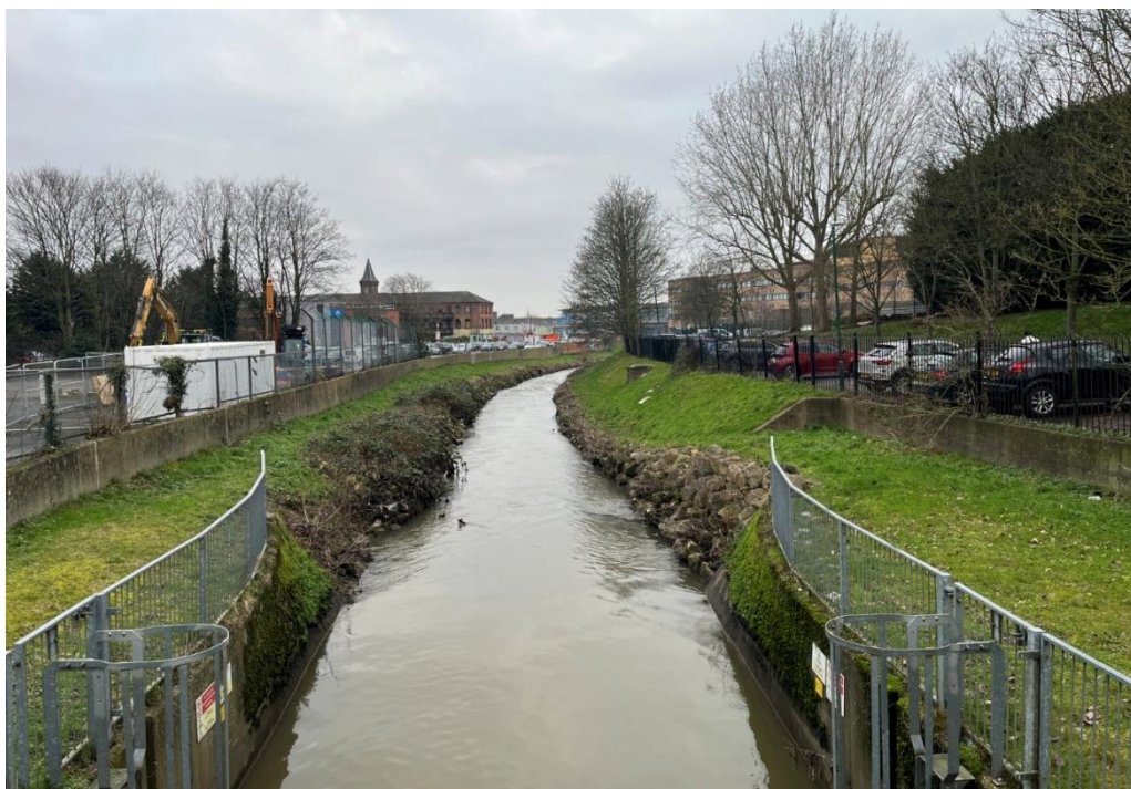
Figure 41: Emerging into area with a concrete flood wall at SK54935 39087 (LB, left of frame) that is beginning to twist and deform. Ideally, any remedial actions for the wall should include ecological improvements to the river corridor. Note the fence on the RB which creates a sense of physical segregation from river; therefore, people aren't able to enjoy and interact positively with the river. The river follows an adjacent cycle path at Hill Side. This section connects with the QMC hospital site (see section in Figure 42). This section is being considered within the River Leen Strategy with options for de-culverting and setting back the existing flood wall to create more space for river restoration, flood capacity and amenity/access improvements.
