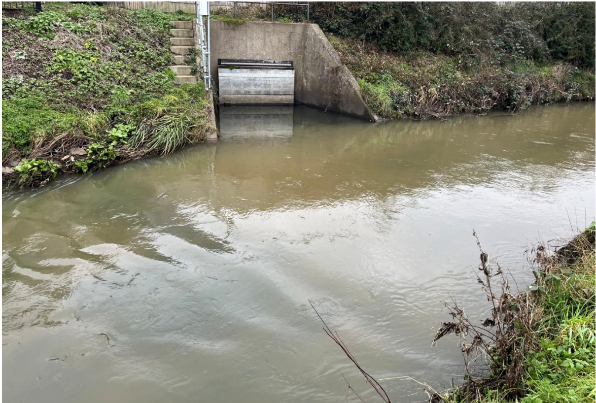
Figure 24: Apparent penstock/flow control and level gauge on outfall on the RB at SK55173 41656 as well as a submerged, low-level weir crest. Exploring the potential to remove or notch this weir is advised. The river then runs downstream through a very straight section adjacent to Bobbers Mill. The channel features grassed flood embankments on both sides and is tightly constrained by surrounding infrastructure (Figs. 25 and 26).
