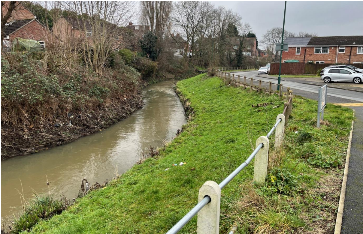
Figure 30: Contrasting vegetation-management between LB and RB, along with extreme proximity of the wetted channel to housing and road.
