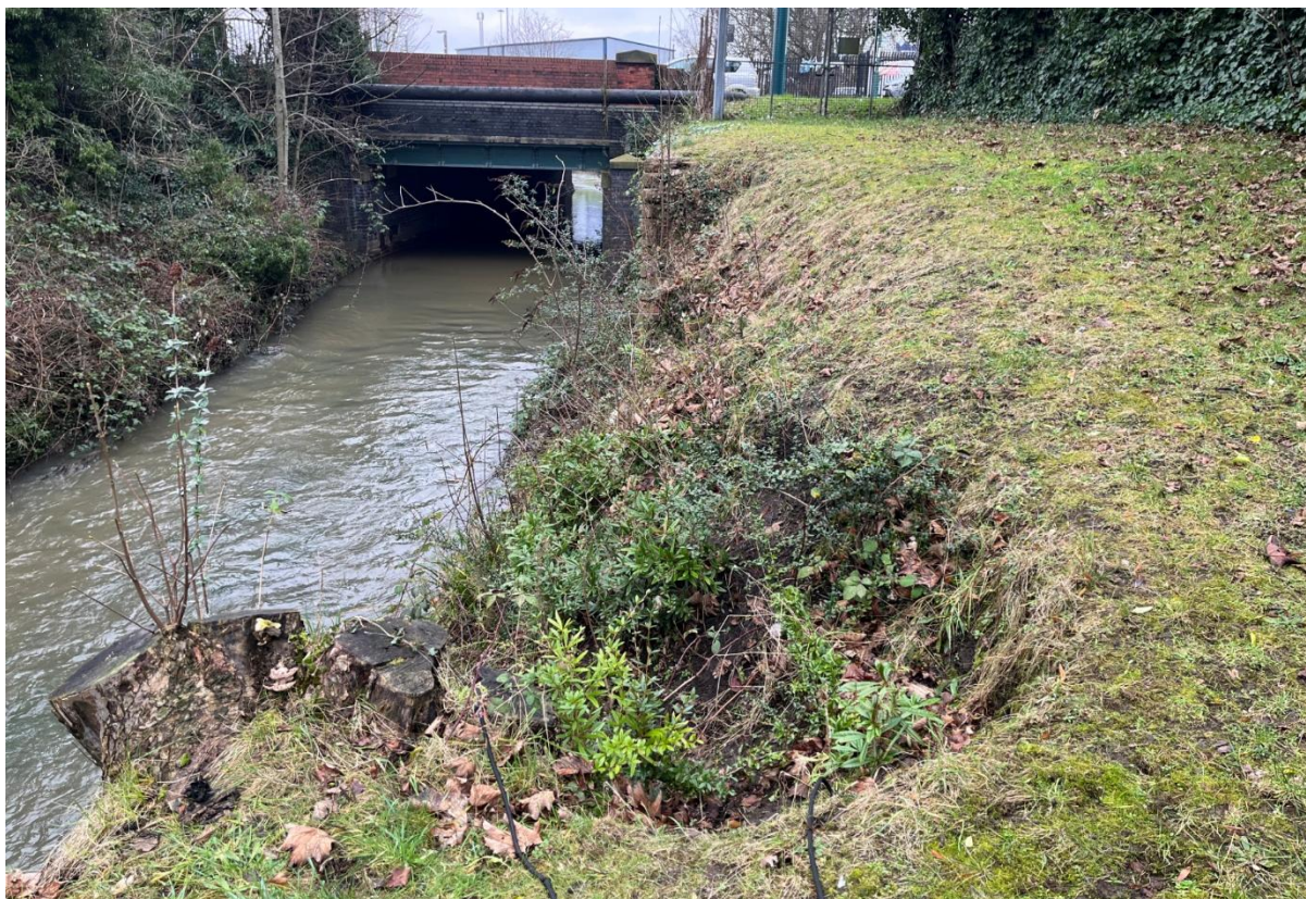
Figure 22: Detail of bank collapse upstream of weir shown in Fig.20.
