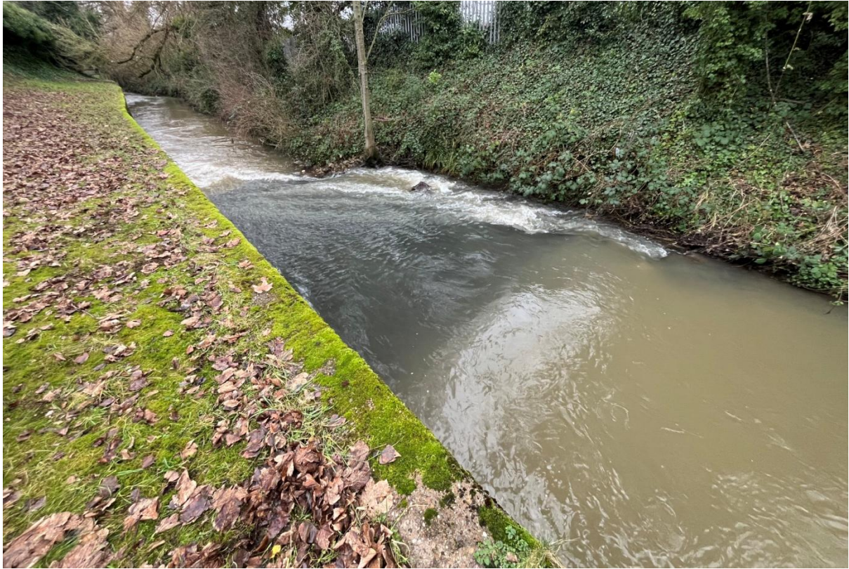
Figure 20: Weir at SK5543041796 downstream of Wilkinson Street could, as a minimum, benefit from hydraulic roughening of the smooth apron so as to create a rock-ramp style fish passage easement and improved habitat. Upstream walls are already collapsing close to the Wilkinson Road bridge, so any head-cut erosion from weir removal would need to be incorporated into the preferred option of full weir removal.
