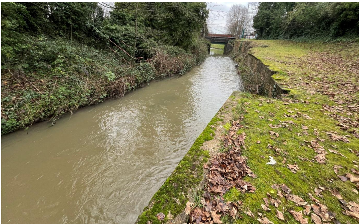
Figure 21: Facing upstream from the weir shown in Fig.20. The wall on the LB (right of frame) is beginning to collapse. Potentially the repair and mitigation of that situation could be used to argue for a weir removal along with appropriate mitigation for head-cut erosion risks to surrounding infrastructure.
