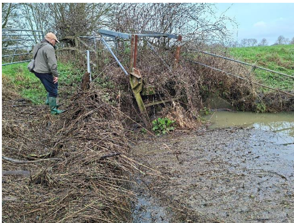
Photo 13. Top-hung tidal gate at the confluence with the Ouse. Functional or derelict? These gates will have a profound impact on the ecology of the lower section of the stream and the species that need to navigate in and out of the system.
