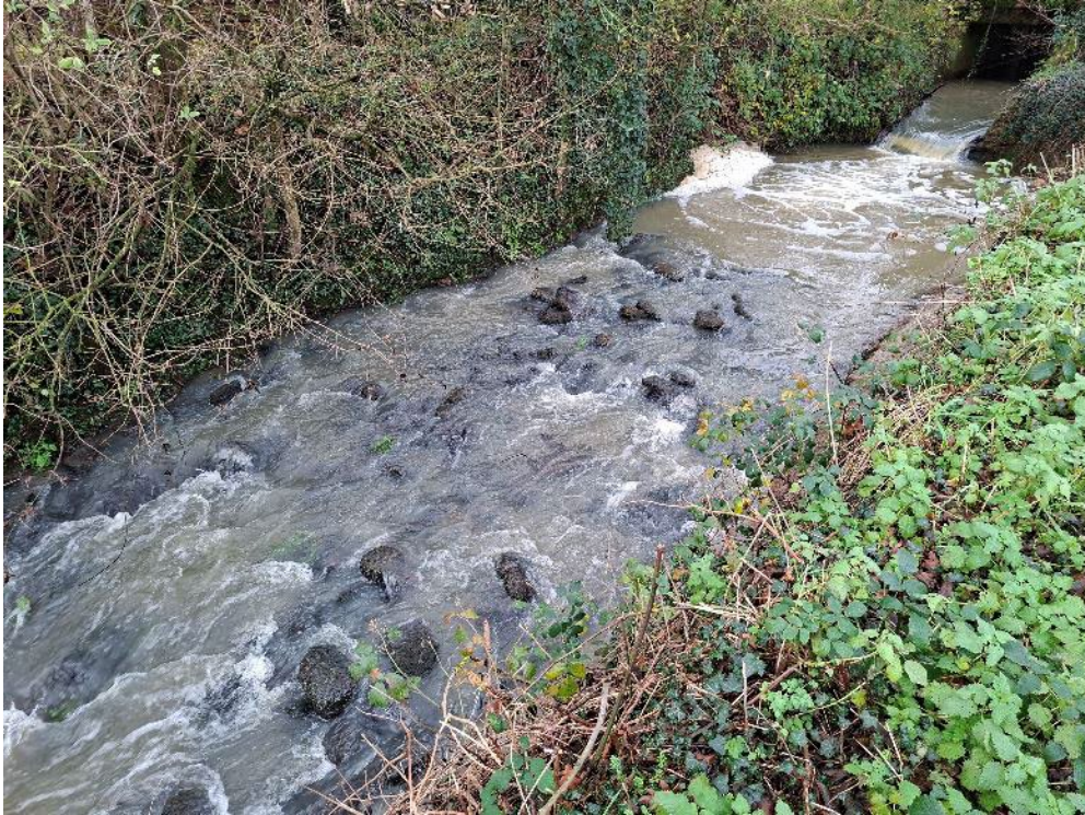
Photo 2. A typical bridge culvert on the Northend stream. These can be difficult for fish migration, but this example looks to have received a pre-barrage of imported rocks, designed to help drown out the invert of the culvert and give migrating fish a better chance of making upstream progress.
