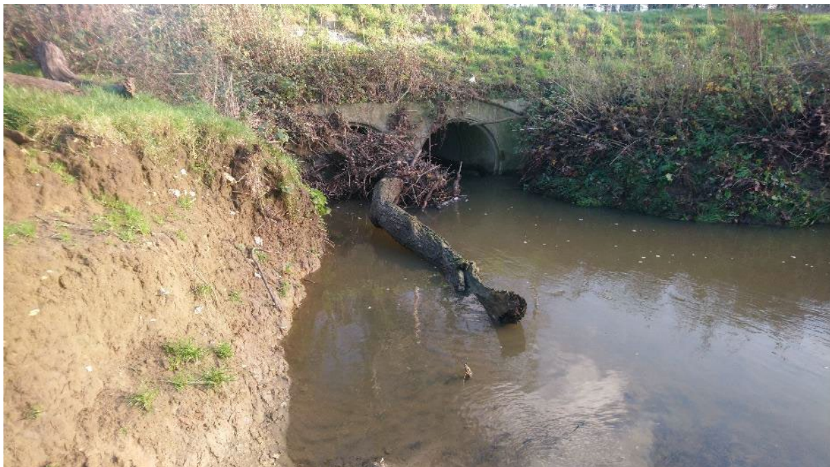
Photo 4. The inlet of a partially blocked culvert bridge, subsequently cleared out by the volunteers.
