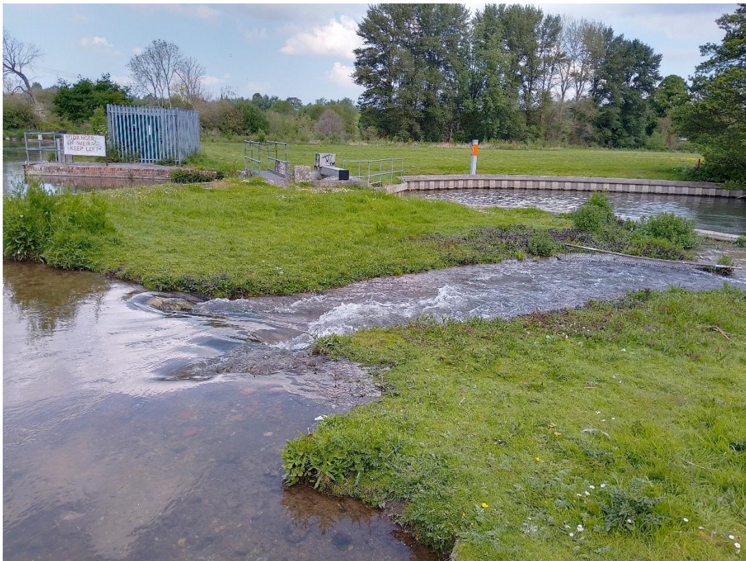
Photo 18 The breach takes a significant volume of water and is increasing in size. This either needs repairing to protect against bank failure near the canal, or could be reviewed for installing a fish passage solution.
