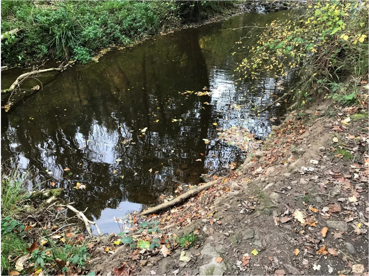
Photo 19 (52.160447 , -2.3717744 ) The erosion into the footpath being forced by the tree stump on the left of this picture. The path has a high-sided bank immediately behind it, so cannot move slightly to accommodate the erosion; it either has to completely relocate into the woods by some distance or further bank failure needs to be prevented to allow the path to stay where it is.
