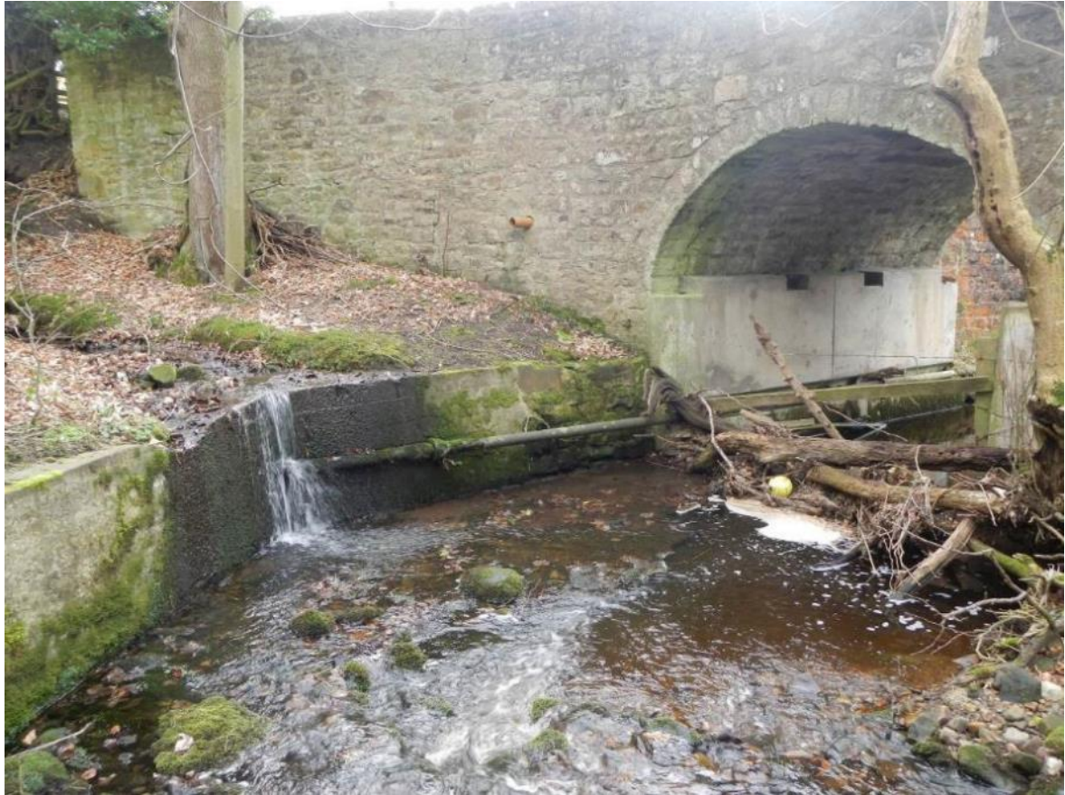
Photo DSCN6318. Although some woody material clearly accumulates against the relatively clear-span road bridge (some concrete footings), the blockage did not appear to be a major fish passage issue.
