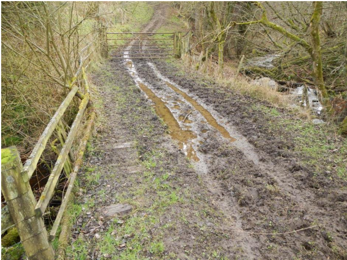
Photo DSCN6247. A track crossing at NY 82894 66096 creates another fine sediment input to the burn, with the track/wheel ruts channelling surface water and fine sediment runoff.
