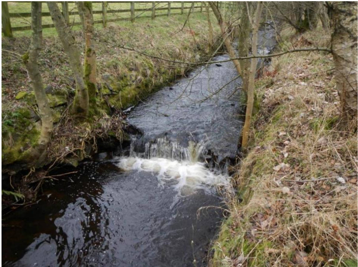
Photo DSCN6325. The burn enters a woodland d/s of the bridge and, for a short distance (NY 82229 64946 and NY 82165 64898) flows within a concrete reinforced channel, with the shallow, uniform flow creating an un-natural impediment to fish passage. The purpose of the lined channel was unclear. At the d/s end, the channel has become undercut and appears to be disintegrating, which is naturalising the channel but also creates a step which further inhibits fish passage.
