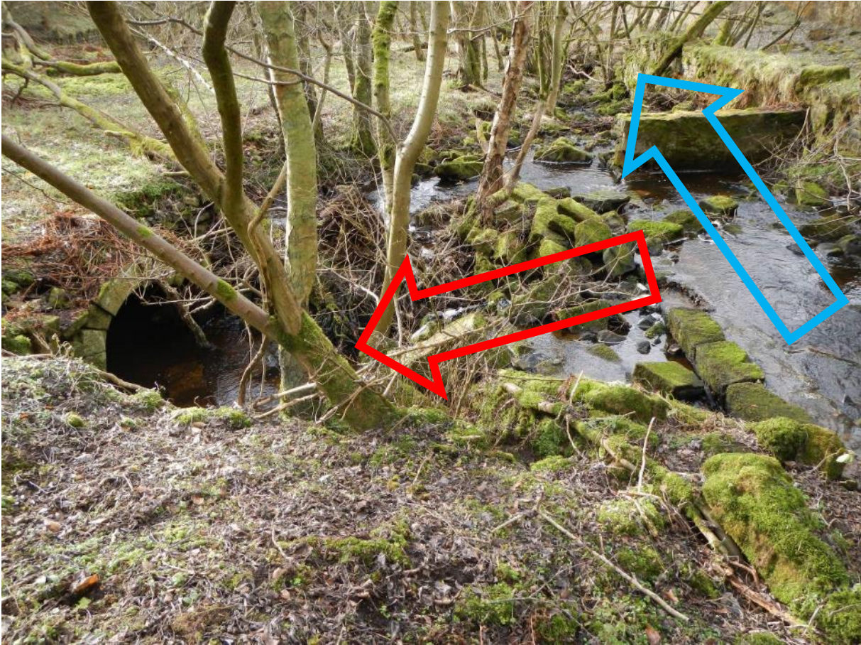
Photo DSCN6254. The offtake at NY 82645 65903, where the historical main channel (blue arrow) loses the majority of its flow to the side channel (green arrow). Neither the original main channel (concrete lined and steep) nor the current main flow channel (underground) could provide adequate fish passage. Major work is required at this site but, owing to the dilapidated nature of the structures and space available, significant improvements are likely to be easily possible.
