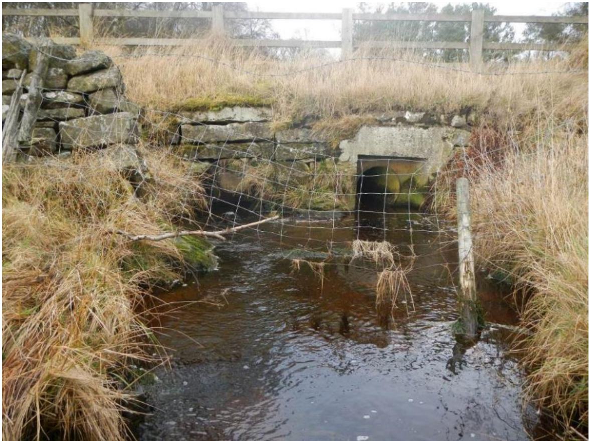
Photo DSCN6225. At NY 82976 66482, the Haresby Lonning (road) crosses the burn, where the burn is piped through two relatively small diameter pipes. While this is far from ideal, the pipes are partially sunken and fish passage at low and medium flows is unlikely to be a major problem. Fluming of high flows may cause some obstruction.
