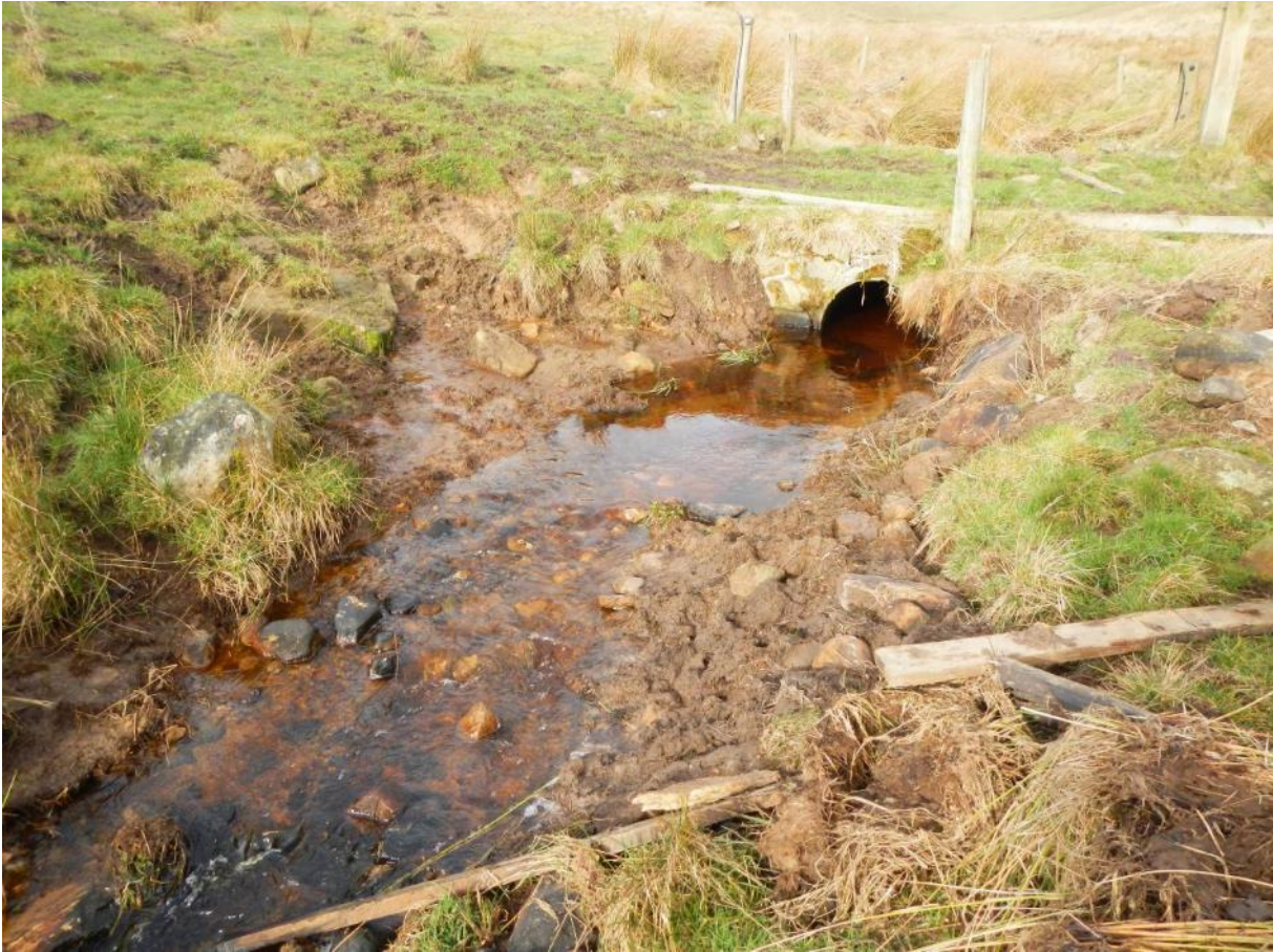
Photo DSCN6191. At NY 82318 67116, a more sympathetically installed culvert creates no obstruction. Poaching and bare bank around the culvert, however, creates a fine sediment input.
