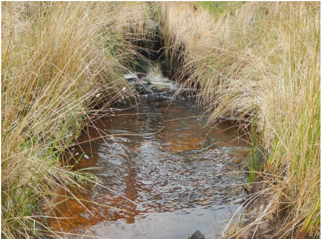
Photo DSCN6190. At NY 82172 67252, a small pipe culvert creates a minor obstruction to fish movement but could have been prevented by simply using a larger diameter, partially sunken pipe.
