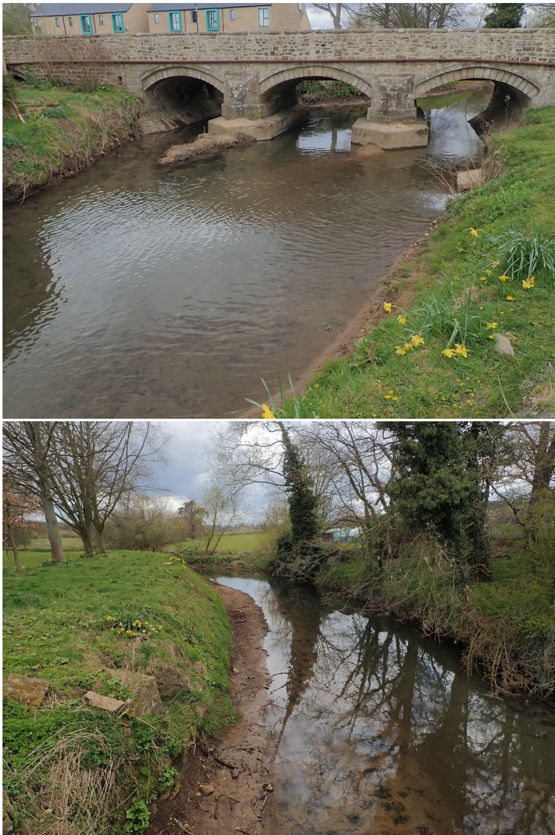
Fig 9. Views d/s & u/s of Gilling Bridge (NZ 18326 05215) of the dredged, trapezoidal channel and the deposits of fine sediment building up in the lee of the buttresses. It was noted that further arches originally built into the bridge had been blocked presumably to allow for development. Reduction of capacity at this man-made pinchpoint clearly increases likelihood of flooding.
