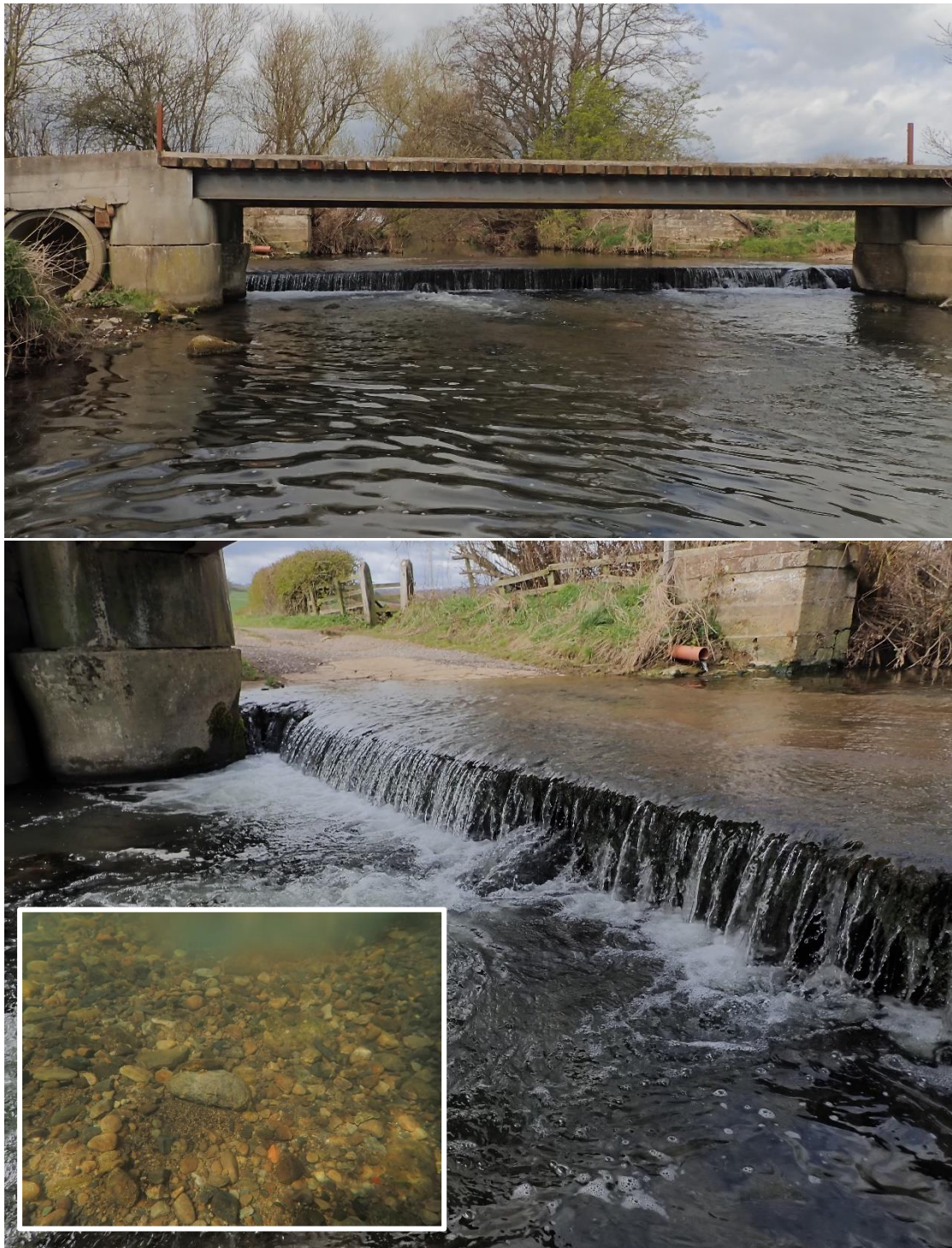
Fig 1. The ford at NZ 19597 03780 marks the d/s limit of GWFF water. It was a complex structure comprising multiple parallel culvert pipes of inappropriate diameter ( \sim 0.5\text{m} ) in a concrete fillet. Several of the pipes were blocked and clearly had been for some time, and all the remainder had debris partially blocking the u/s side contributing to the impounded reach which extended for \sim 50\text{m} u/s. A considerable barrier to fish passage and sediment transport, especially considering the clear span bridge adjacent. Insert highlights where flow energy was concentrated, the gravel could be kept clear of fines.
