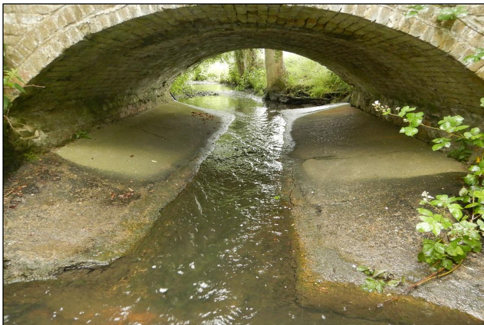
Pic 10 – If fish reach the bridge in low flow, they have very shallow water to swim through because the easement was not finished to the crest height of the obstruction. In high flows the water velocity and smooth bed will make it challenging for most species to traverse. Passage through the bridge could be enhanced by the installation of stones fixed to the base of the bridge to increase its roughness whilst creating small pockets of calmer water to aid resting. Similarly, flow baffles could be attached. See example of fish passage easements in Recommendations.
