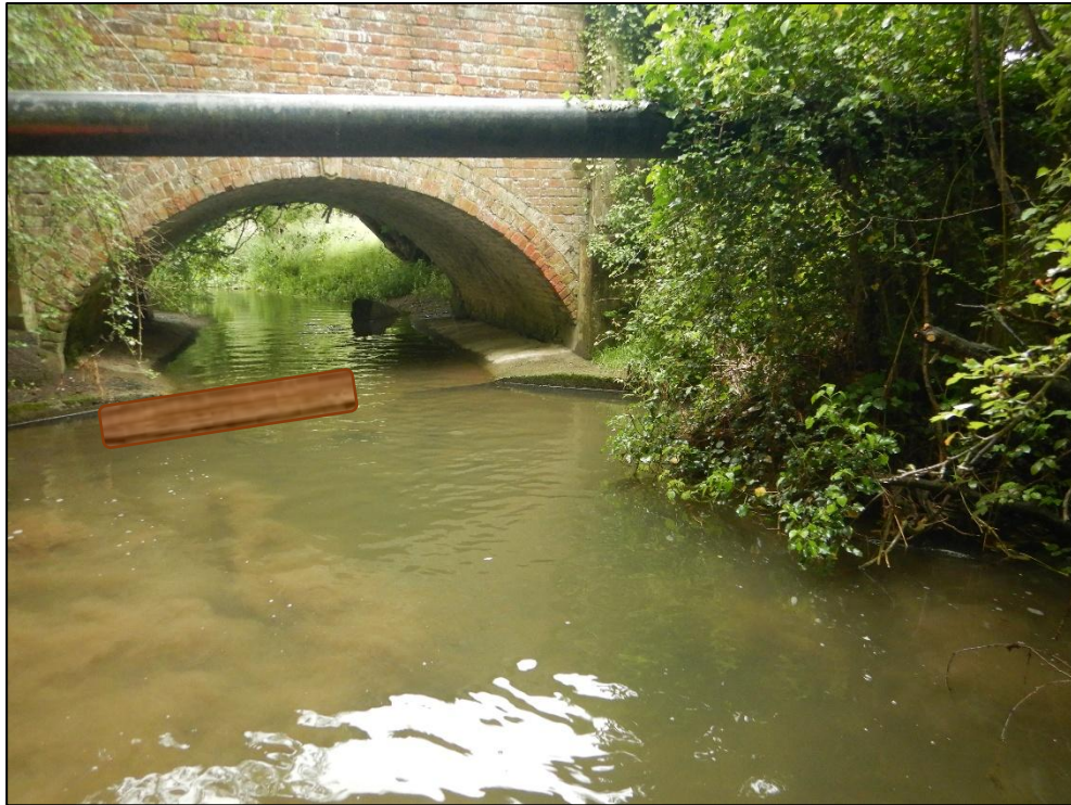
Pic 23 – Access for fish through the bridge is possible at all water levels. The bridges shown in pics 10 & 12 should be like this and could be so with appropriately installed rock ramps, which actually drown the invert of the structure. Note the high fine sediment load disturbed as soon as the pool was entered. It is degrading the habitat. If it were not for the excessive fine sediment this pool would offer good trout holding potential given its low trailing cover. The positioning of a flow deflector (note illustration) could enhance the main flow pathway to the trailing cover.
