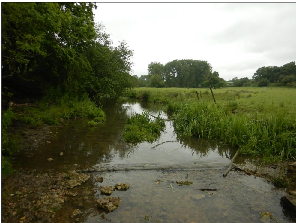
Pic 38 – Once again a weir removal has removed most standing blocks to lower the upstream impoundment of water, but by unnecessarily retaining the foundation a shallow weiring effect is still present. Unless there is a need to retain the upstream pond habitat, the weir's complete removal should be sought as in low flow conditions it still presents a barrier to fish (such as bullhead).
