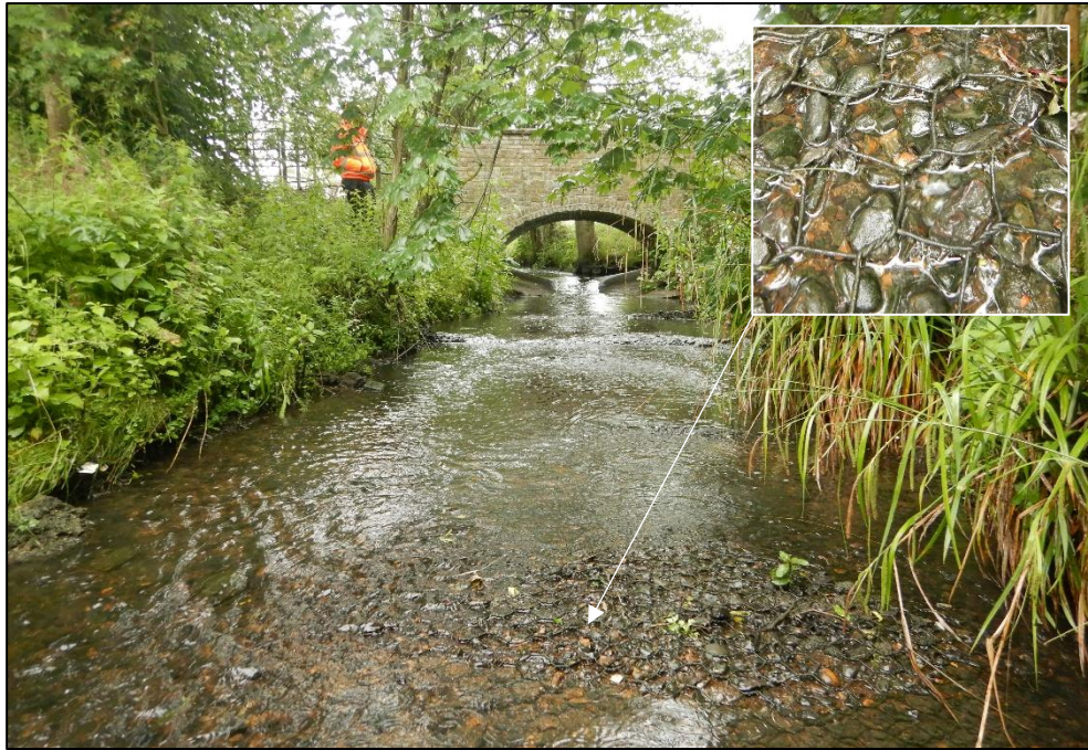
Pic 9 – A rock ramp has been installed to raise the bed level of the Stevenage Brook, allowing fish to swim up and through the bridge. The rock ramp was constructed with stone held by wire mesh, which is now exposed making it vulnerable to damage and possibly hazardous to animals. The original design for the rock ramp should be revisited, if it was meant to be capped with gravel then it should be topped up. If not, then presently there is little cover for fish moving through this reach and the original designer should be asked about measures to improve the approach. Caution should be had at any measure that could potentially damage the mesh holding the stone.
