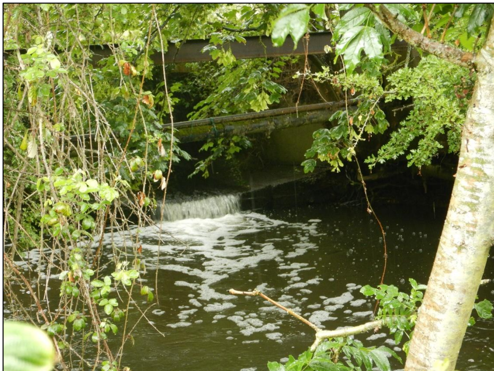
Pic 12 – Approximately 80m upstream from the rock ramp easement another bridge was encountered. The drop from bridge base to water was ~0.15m. It may have been may have been accentuated by the low flow conditions, but it still presents an obstruction to the movement of fish and river substrates. Access through the bridge should be enhanced by the addition of stones set into the base of the bridge, but that does not address the problem that the bridge poses to the river corridor.
