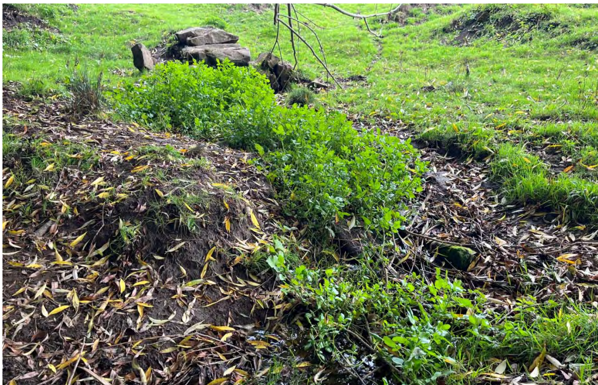
Figure 21: Emerging at the piled stones in the background, an orange coloured discharge trickles towards the river.
