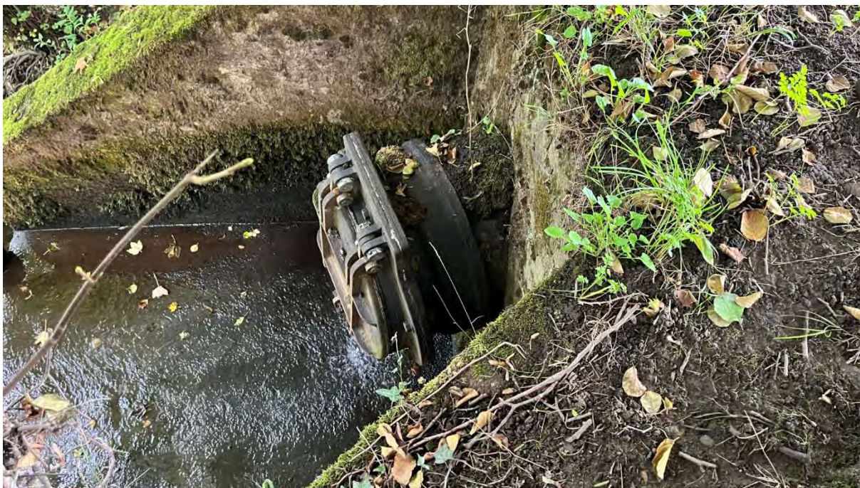
Figure 10: Outfall that is apparently in use. At the time of visit this was not showing gross signs of pollution.
