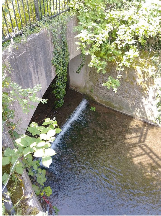
Photo 9. The downstream end of the culvert with the footbridge over the top of it, a small step in concrete bed level creates further fish passage issues.
