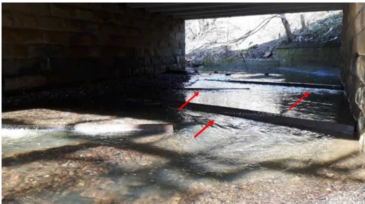
Figure 5 Alternatively, a series of low baffles can be installed in a culvert to create depth and flow conditions allowing fish to pass through at low flows (red arrows highlight the baffles)
