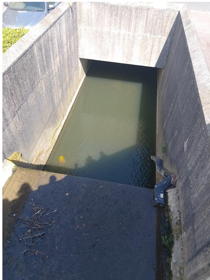
Photo 12 The large vertical drop and next culvert – right hand channel. An elver pass has been installed to the side of this.
