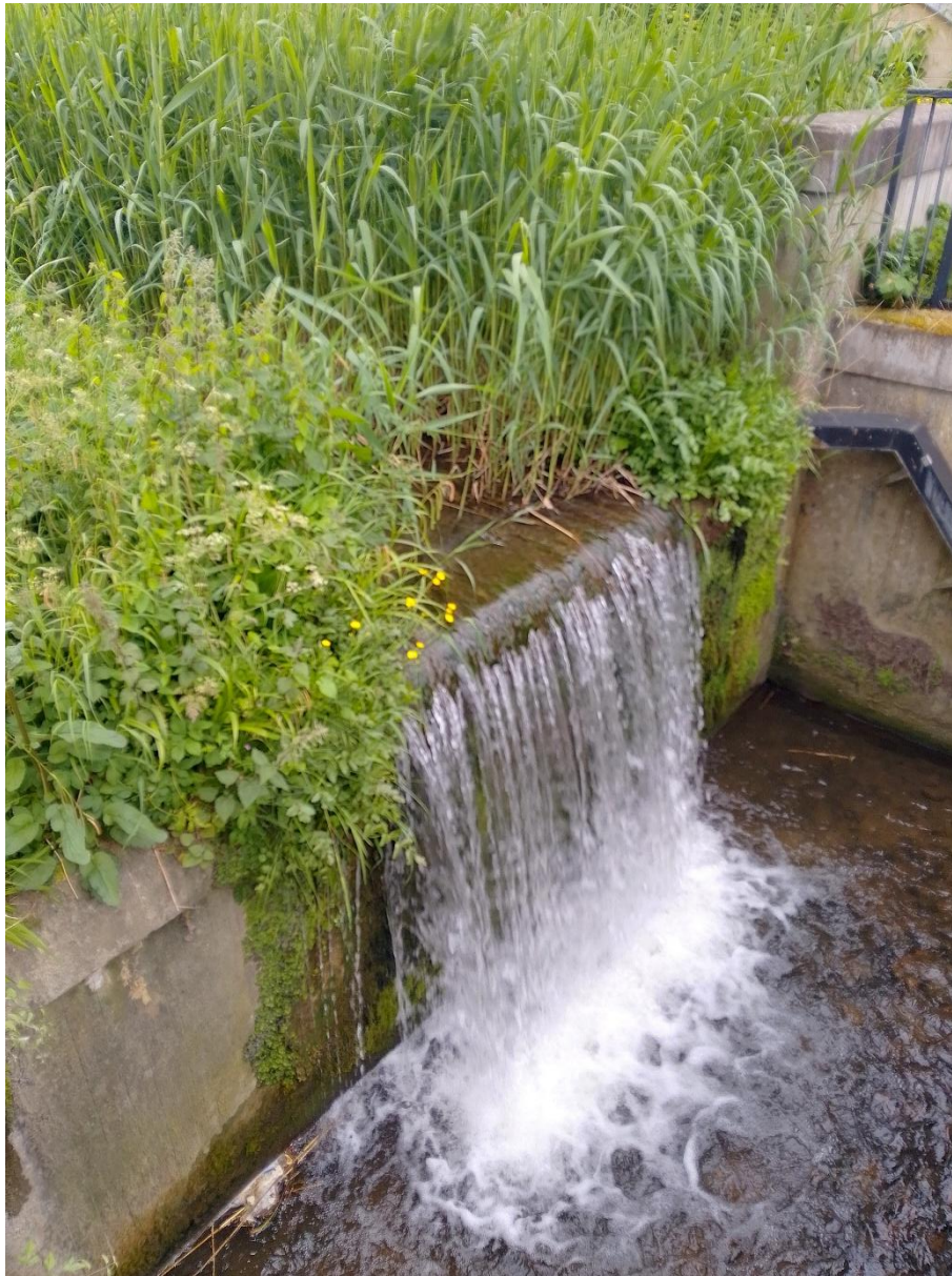
Photo 15 The vertical drop at the end of the St James Walk 'overflow' channel. Another elver pass has been installed on the far bank.
