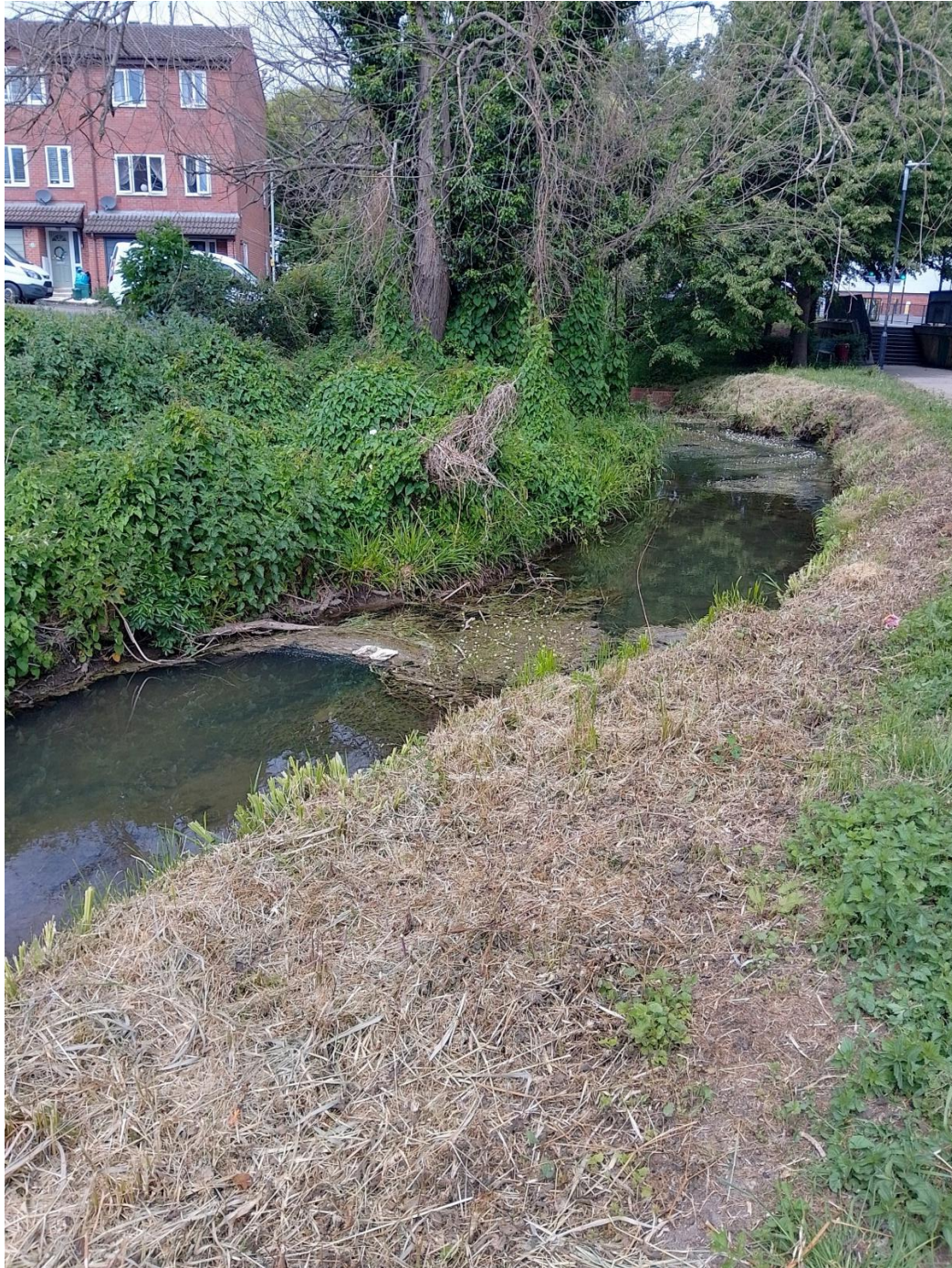
Photo 22 The end of the section of Chelt reviewed at Gloucester Road. The end of the channel that can be seen in the middle distance becomes quite constrained and a small brick wall interacts with the channel. This should be reviewed to avoid any influence on flood water being backed up by the constraint here.
