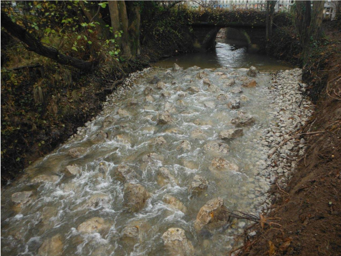
Figure 7 Example of a rock ramp. It could be possible for the concrete in the overflow channel between Honeybourne Way and the weir to be chopped out, reformed and a rock ramp installed across the gradient between the Chelt downstream on the road culvert – buried underground service cables and pipes allowing. Alternatively, a technical fish pass could be investigated, but these are very expensive to install and need maintenance. Baffles at the entrance to the culvert may be required to maintain water depths and velocities to enable fish passage. It may be a variation on this solution could be used at the top of the overflow channel to get fish up to the Waitrose car park culvert.
