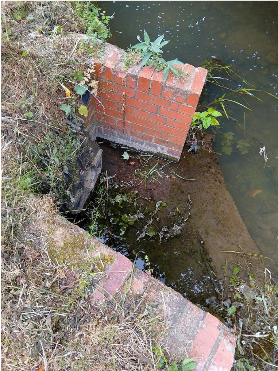
Photo 18. One of two adjacent storm overflow drains (51.903289 , -2.0874793). What gets discharged to the watercourse from these drains is always a big concern. Obtaining a services map of pipework to review the likely inputs will help understand water quality impacts to the Chelt. GORC can also actively monitor upstream and downstream during periods the pipe is running. Concerns would be contents of road run off (microplastics and pollutants) and misconnections in residential properties (washing machine phosphate input). Mapping features like this and engaging the Council may provide opportunity to break these out (space provided) and run through an urban sustainable drainage system feature (SUDs – e.g. swales, retention pools etc) to allow the water to settle out fine sediment and contaminants a little before reaching the river. Examples such as the 'Outfall Safari' highlight where community groups have mapped issues before: https://www.southeastriverstrust.org/projects/outfall-safaris
