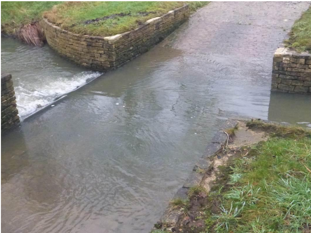
Photo 17 (52.983966,-1.6383241) Ford: passable in certain conditions, but an obstruction to fish dispersal and migration. Ideally this would be replaced with a clear span bridge or appropriately oversized sunken culvert, alleviating the issue for fish movement and also improving access.
