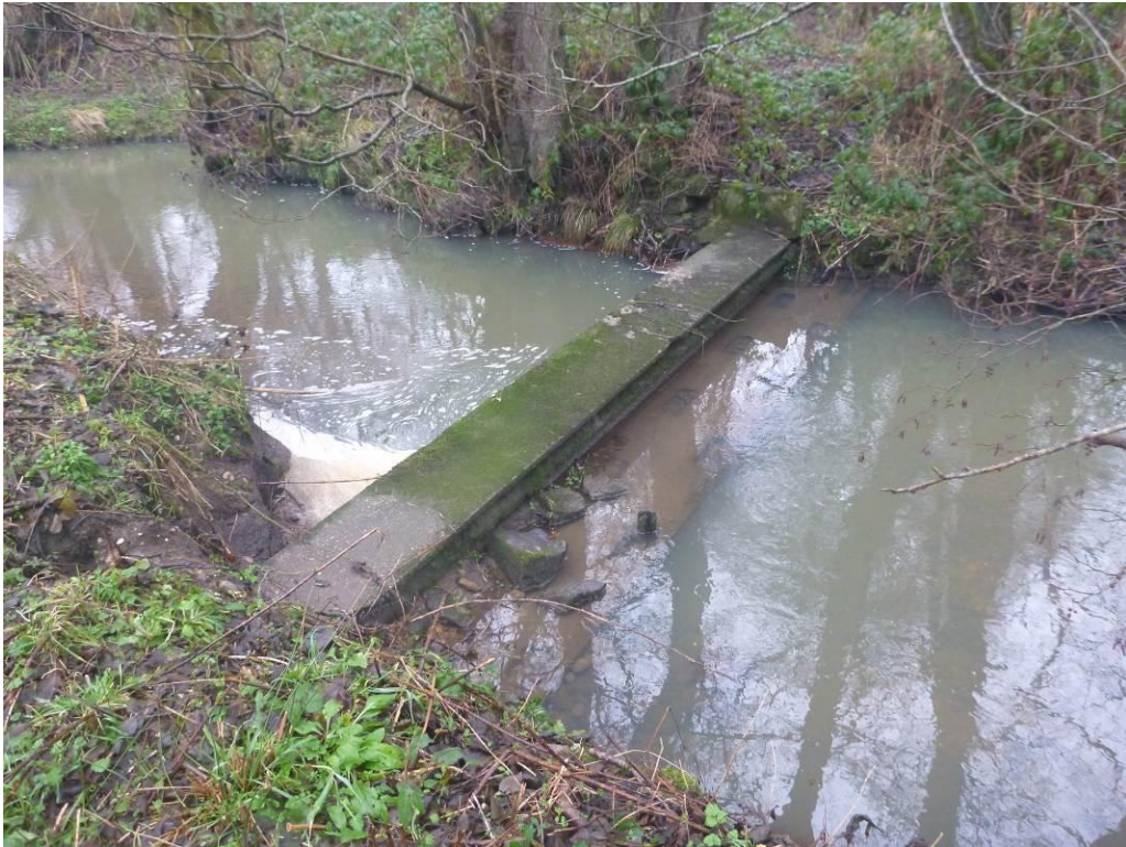
Photo 54 Partially breached weir.
