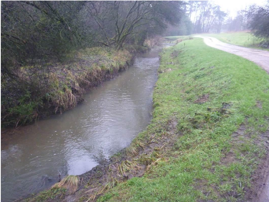
Photo 22 Hard bank protection (rock rolls at the toe) has stabilised erosion alongside the track, but the issue stems from the historical realignment of the brook from its likely natural course into the straightened channel, which also lacks natural habitat features.
