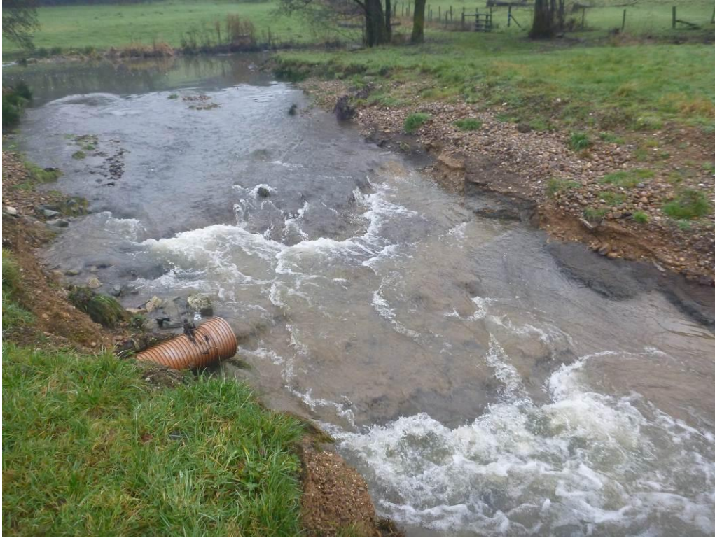
Photo 12 Upstream end of rock ramp showing loss of introduced bed material (bare clay).
