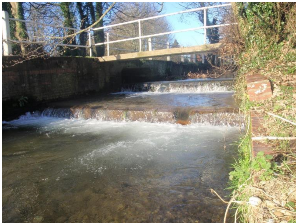
Retrofitted fish passage improvement: new pre-weir (foreground), raising water levels at the existing weir (background) with a radiussed notch in each.
