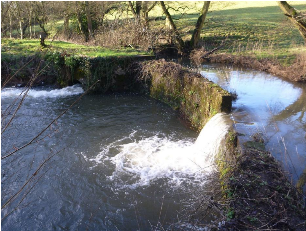
Figure 27 Weir prior to notching (in 2016) during high flow conditions. During low flows, water would pass only through the far sluice at high velocity (preventing fish passage).
