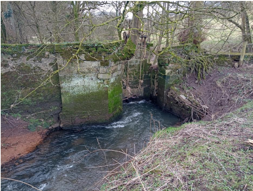
Figure 23 Dilapidated sluice – this is not a barrier to fish passage as long as it is not blocked.
